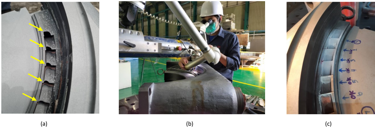
Fig. 15. (a) Eroded and corroded blades of turbine nozzle; (b) Laser welding repair; (c) Repaired blades after grinding and liquid penetrant testing
